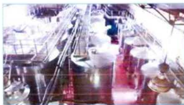
Wine Fermentation Tanks
